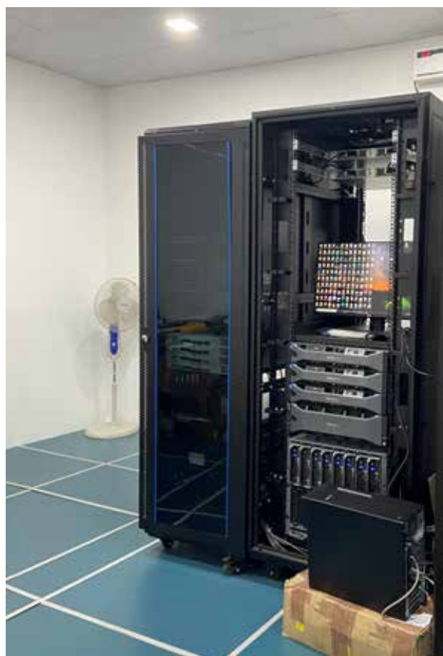
Figure 17 Server Room (Source Authors)
