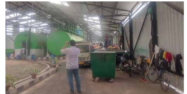
Figure 8: Bio-methanation plant at New Town Kolkata Source: Authors
