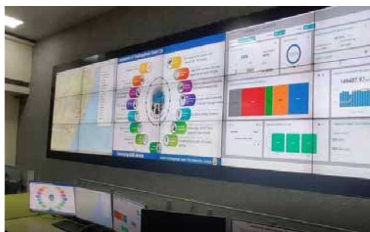
Plate 05: Dashboard with various sub-systems in ICCC
