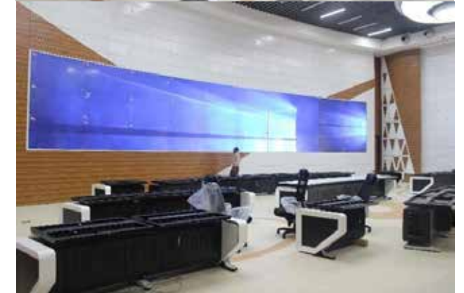
Figure 9 : Integrated Command and Control Center (ICCC), and Supervisory Control And Data Acquisition (SCADA) Center
