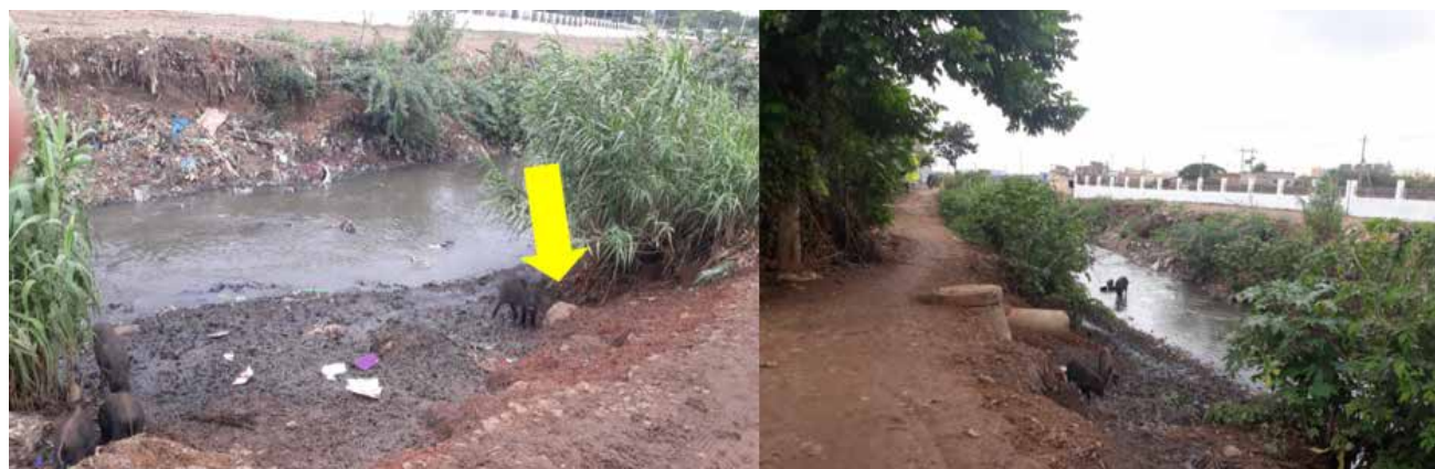
Image 1: Discontinuity and utility pipe issues in storm water drains.
